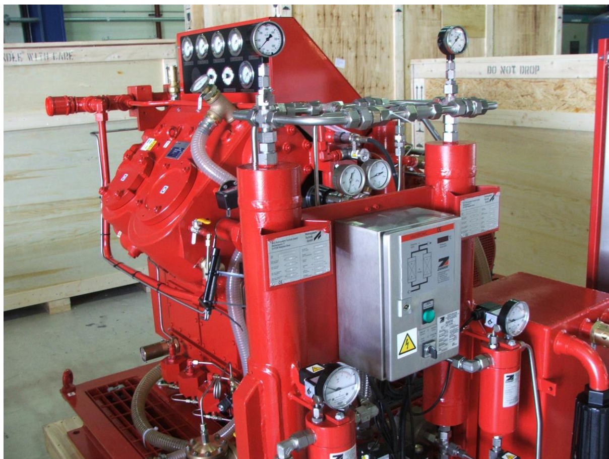
Typical installation, Drilling Rig North Sea
